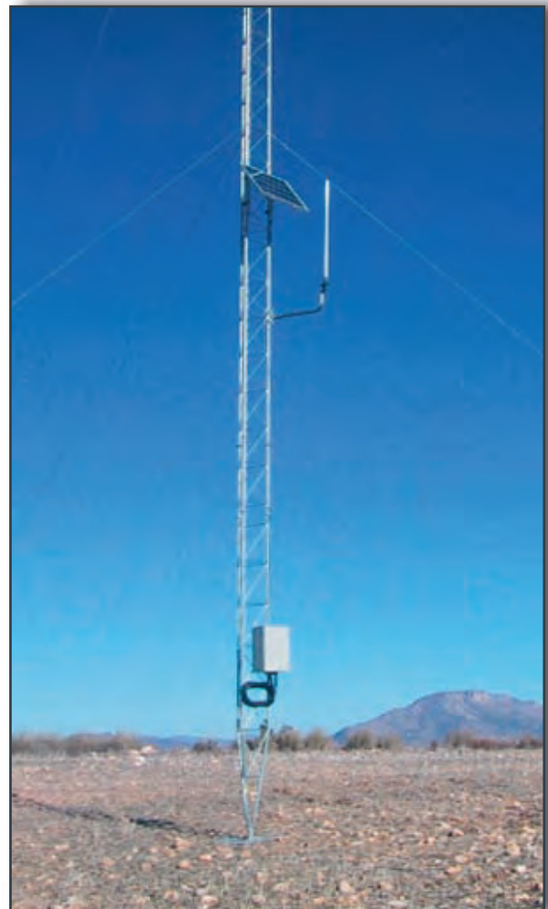
METEODATA-3000C Data Logger, a high gain GPRS transmitting antenna and a Solar Panel, mounted on the met tower
